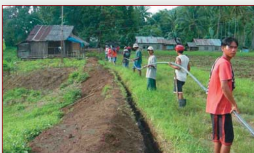
Laying of pipes for water supply – a joint Company and local villagers effort
