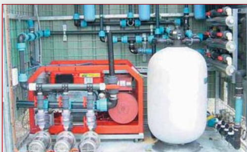
Water purification system and pumps
