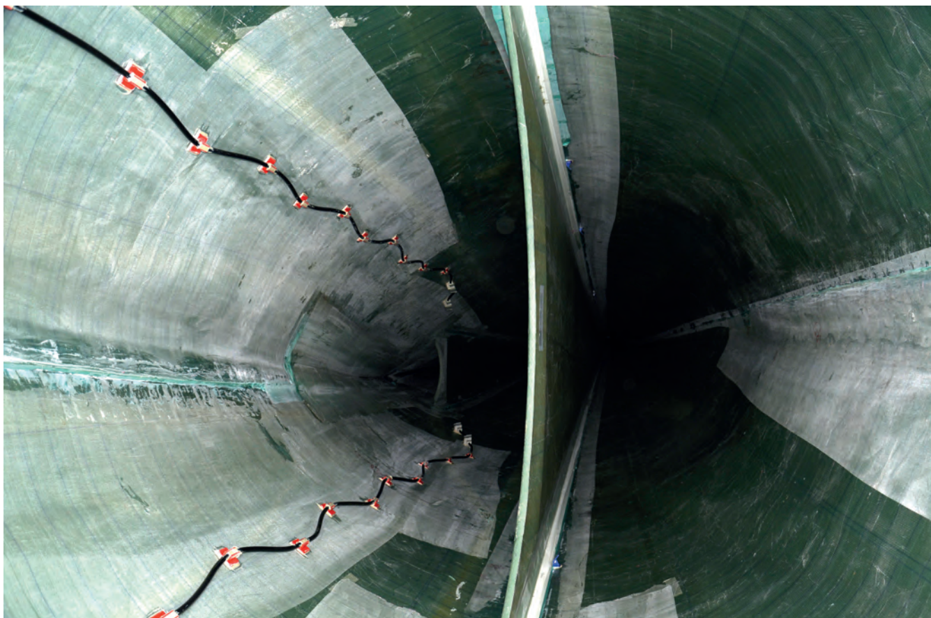
Lightning protection system, Douglas West blade
