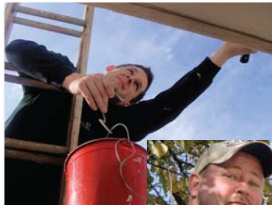
Painting the Upper Valley Turning Point building for the Second Wind Foundation
