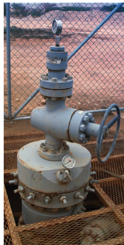
Above: Damis (Block S-1) Yemen – An Nagyah Oilfield: Wellhead.
